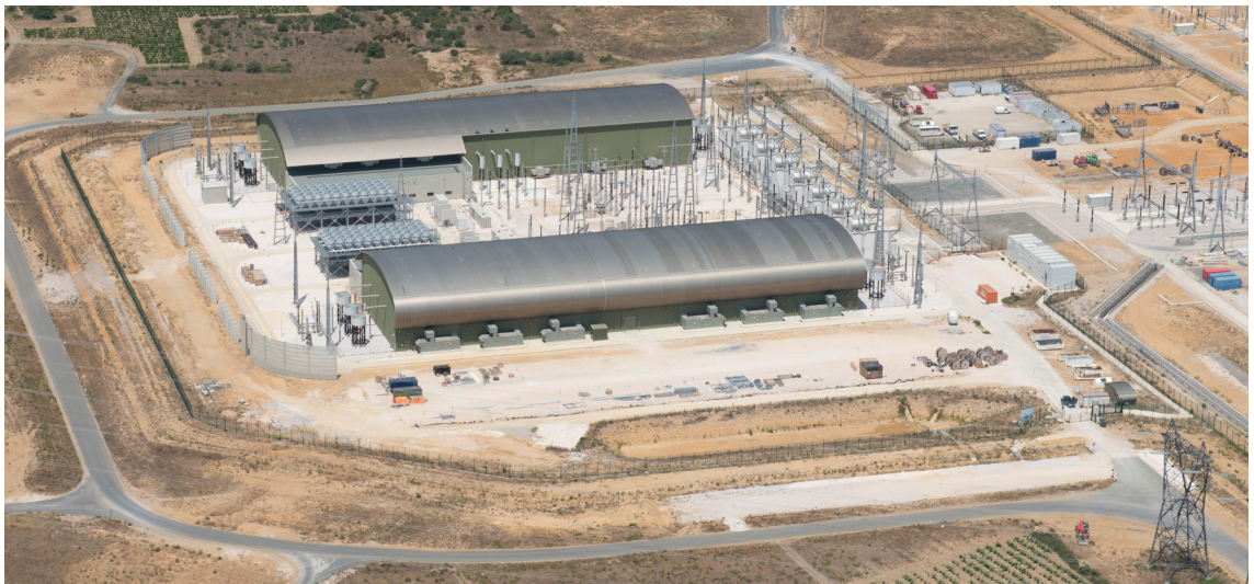
Baixas converter station
